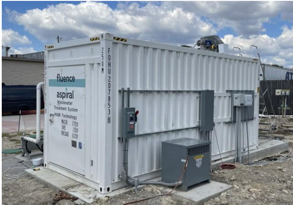
Containerized Fluence Aspiral MABR treatment system installed at Pilot Travel Center 1140
